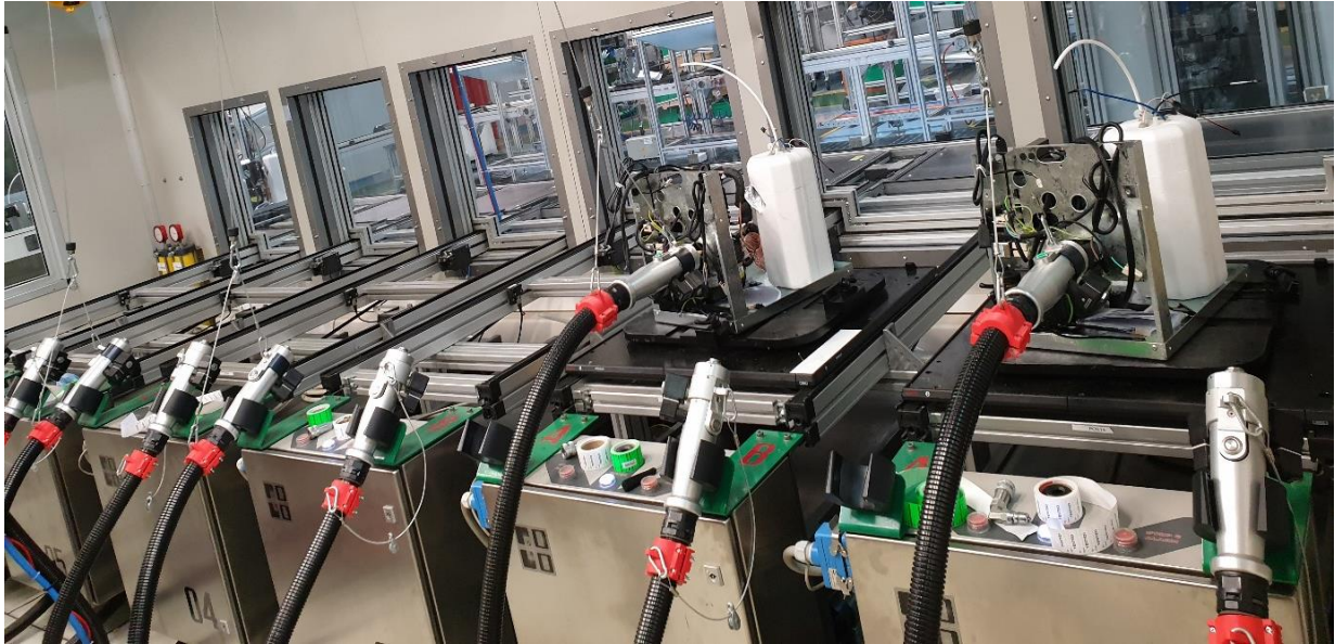
Refrigeration Charging Stations
